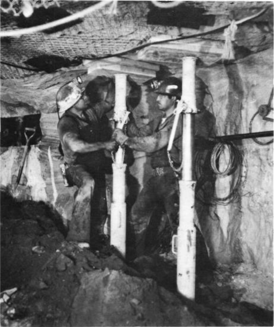
Miners are installing hydraulic roof jacks for temporary support of the roof of a working place. Nets (on roof) and mats (on wall) are installed to prevent falling and slabbing rock. They are held in place by roof-bolts. Photo courtesy of Department of Energy.
